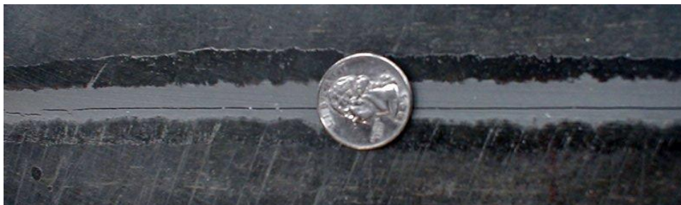
Early, Minor Separation Void – No maintenance generally required
