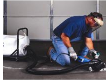
Portion of existing filler is removed Using a dustless joint cleanout saw.
