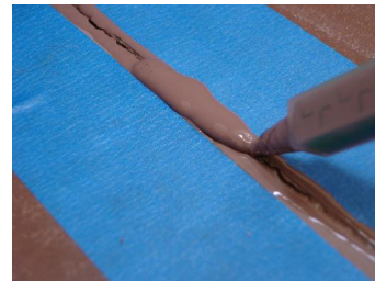
Multiple applications of the filler may be required as seepage occurs.
