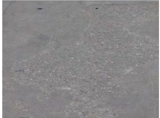
Closer look at deteriorated area
