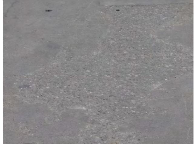
Closer look at deteriorated area
