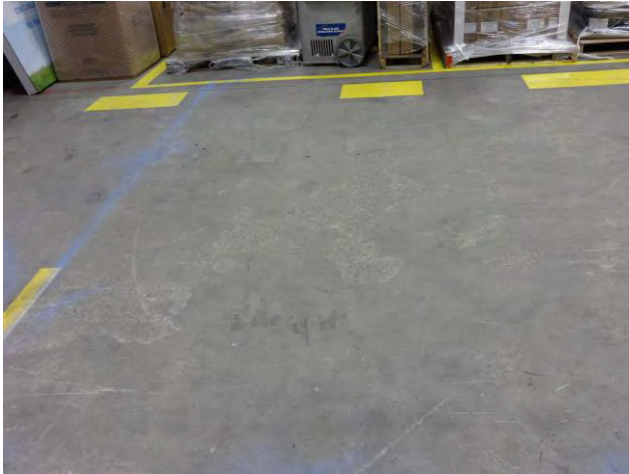
Deteriorated concrete needing to be resurfaced.
