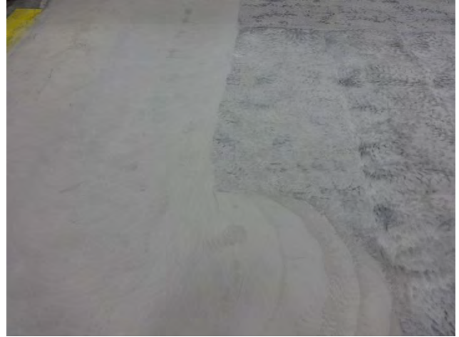
Close up of ground AH HDR
