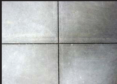
Unfilled At Construction Phase
